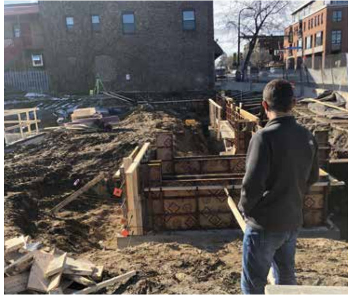
The construction site in February. To learn more about the new Family Tree Clinic or to donate, visit PowerToBuild.org
